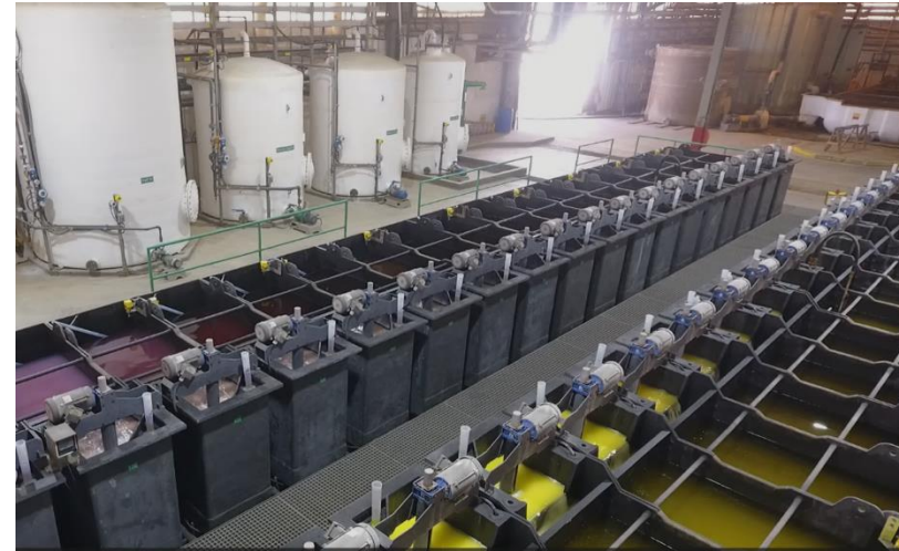
Existing solvent extraction ("SX") circuit at the White Mesa Mill producing NdPr in 2024.
